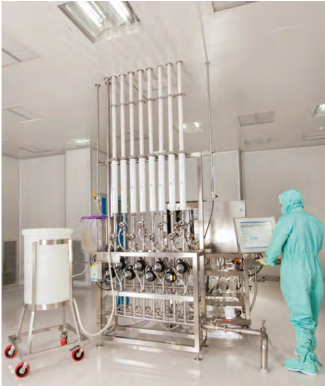
Figure 7. Buffer distribution skid in process room, with flexible hoses directly connected to chromo system and to drum bag for filling.
