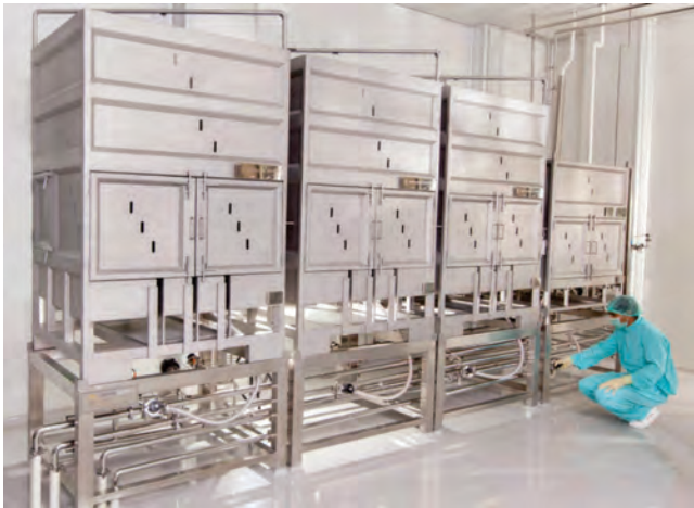
Figure 5. Palletank skid for buffer storage with stainless steel piping headers for filling and distribution, located in buffer preparation room.
